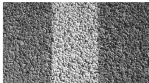
Fig. 8.15—Painted lines visible on pervious concrete pavements.
