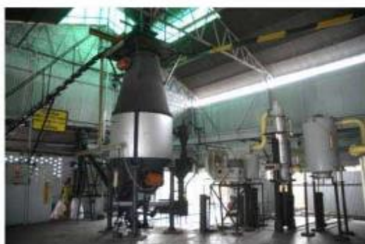
Rice Husk based 250 kWe Power Plant, India
